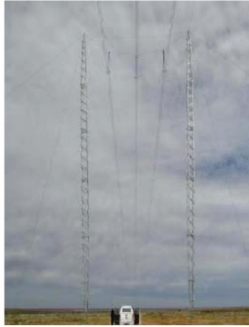
400kV 529A Cross Rope Suspension Tower Max Height: 43m Width Top: 35m Width Bottom: 27m
