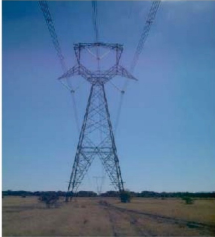
400kV Transposition Tower Self-Supporting Suspension Max Height: 40m Width Top: 17.2m Width Bottom: 9m
