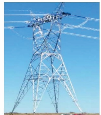
400kV 517E Self Supporting Strain Tower Max Height: 35m Width Top: 22m Width Bottom: 16m
