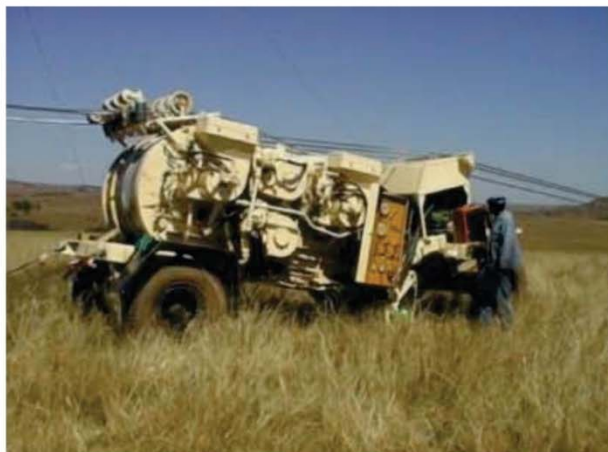
Typical example of tensioner station
